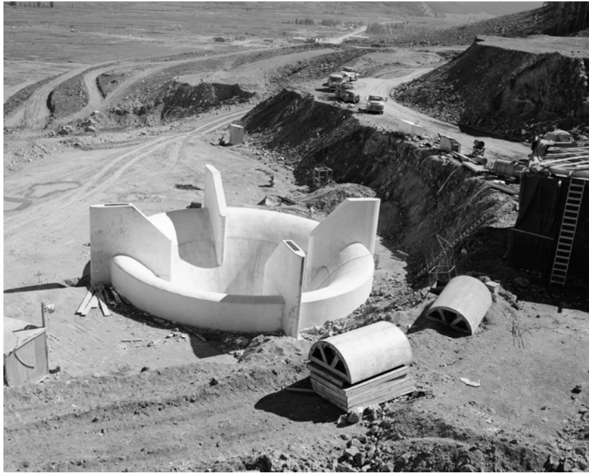
Crews work on building the reservoir’s “Morning Glory” spillway, which discharges water into the Blue River downstream of the dam.
